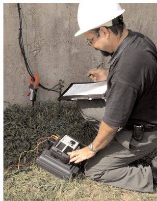
Using ART method with the DET3TC to test commercial ground without disconnecting the system
